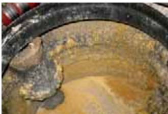
Grease deposits in lifting and pumping stations
