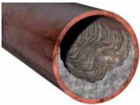
Grease deposits in piping
